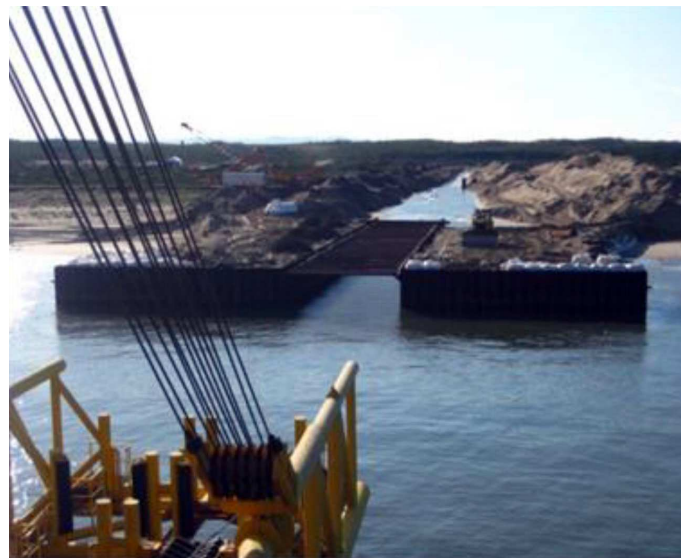
Fig. 10.2-4 Cofferdam for pulling of pipeline on shore at the Kirinskoye field, Sakhalin Island
